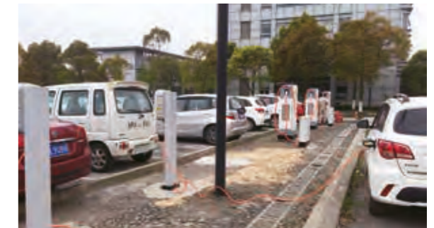
A new energy vehicle being charged with the charging pile installed near the Pudong Service Building of Air China's Shanghai Branch
